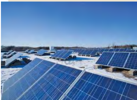
Photo voltaic panels provide active solar energy generation.
