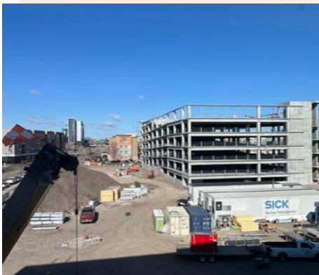
Construction of Phase 2 of the SICK technology campus looking at the parking structure, April 2025
